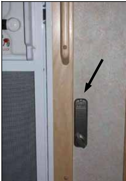
Interior view shows lockset. Note that the lockset is installed in the wall and not in the door.
