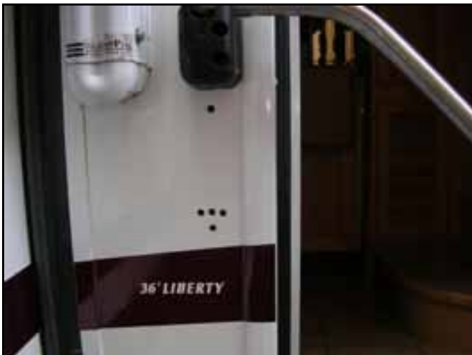
Holes from exterior
