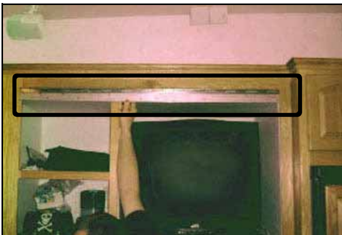
With the left cabinet door removed, I then installed a heavy-duty continuous "piano" hinge at the top.
