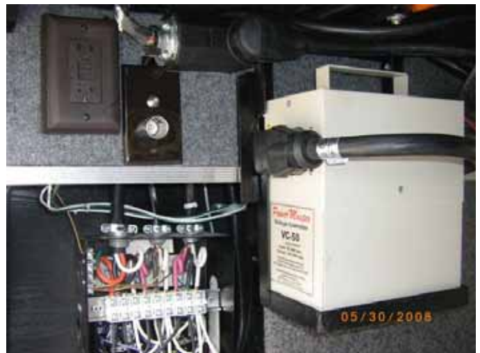
Autoformer box rests on a metal base which is anchored to the structural framework above.
