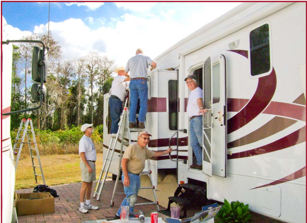
Looks like an old fashioned barn raising, but it's actually a bunch of Tetoners replacing slide gaskets. Helping Joe Betz #130 are Tom Wilby #1450, Dennis Inman #1184, Jeff Engel #316 and Jerry Yoesting #1376 in Clermont (near Orlando).
